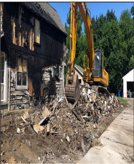
Dominion Energy has had multiple crew members on the scene since the explosion at a house on East 57th Street in August 2021. It is required, according to spokesperson Neil Durbin, to conduct an investigation of the service line and file a report with the Public Utilities Commission of Ohio.
